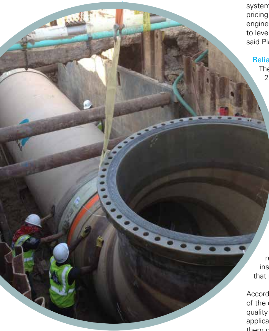
A 72-inch flange was manufactured to tie into a 72-inch steel flange.
